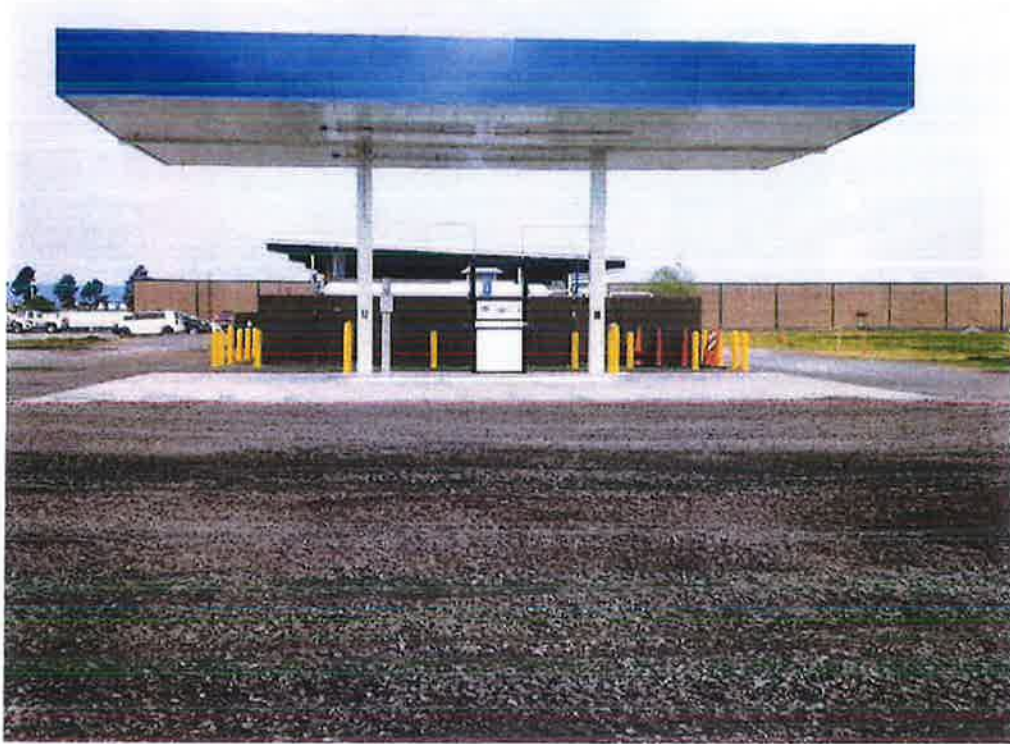
Fort Smith Transit CNG Fueling Station
